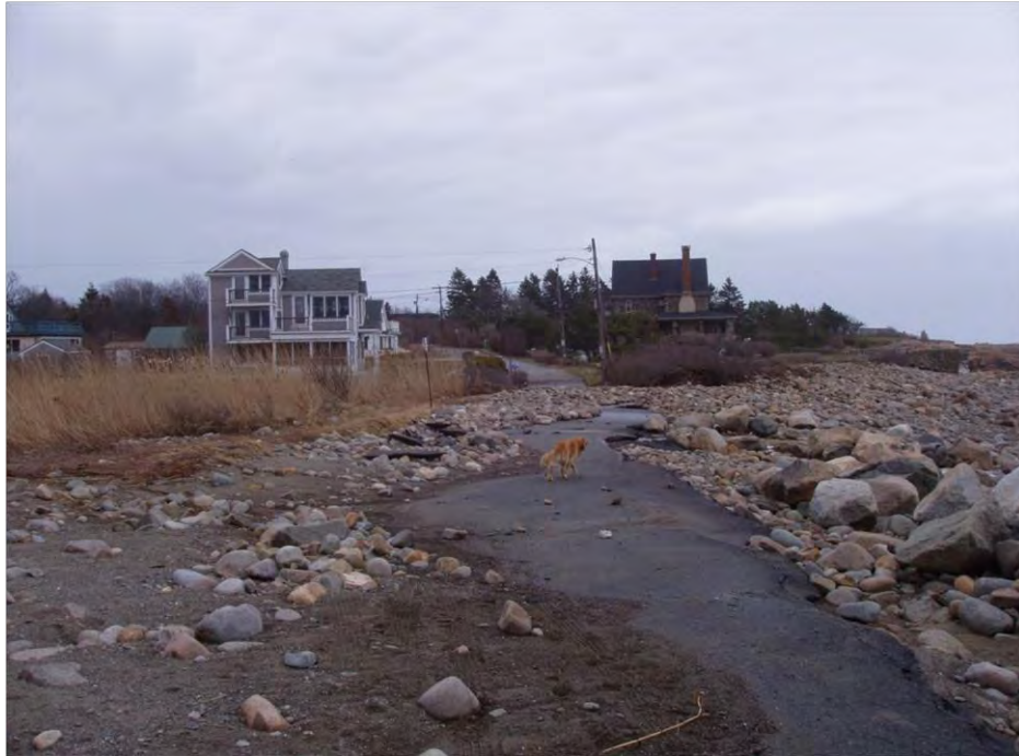
Photograph 4.5. Damaged pavement and overwashed sediment after a recent storm on a barrier beach. Photograph courtesy of Eric Hutchins, National Marine Fisheries Service.
