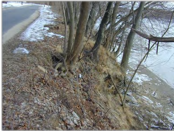
Photograph 2.18. Coastal bank with vertical scarp. The erosional scarp on the side of the bank indicates that this coastal bank is acting as a sediment source, while also maintaining its ability to act like a vertical buffer through its height.
