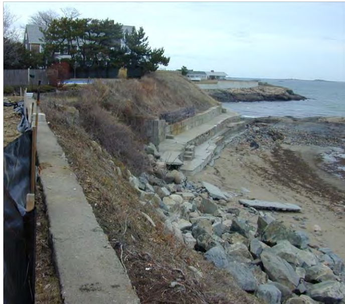
Photograph 4.6. Pre-existing riprap on coastal bank and coastal beach. The rocky intertidal shore can be seen in the distance.
