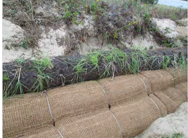
Photograph 3.1. Coconut fiber rolls used to stabilize the toe of a coastal bank. These rolls (some of which were wrapped in natural fiber blankets) were later covered with sand and planted .
