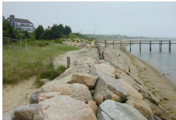
Photograph 1.9. Coastal dune with coastal engineering structures. Foreground: coastal dune landward of rock revetment. Background: coastal dune and beach landward of a deteriorated bulkhead.
