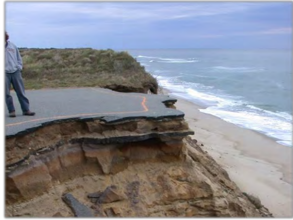
Photograph 2.17. Destabilized coastal bank. The construction of, use of, and stormwater runoff from this pavement has contributed to erosion and destabilization of the top and face of the coastal bank, yet due to its significant height, this bank still acts as a vertical buffer. This bank also provides sediment to the adjacent beach.
